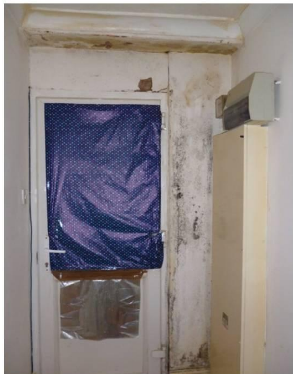
Sadly, an all too typical example of the type of poor property conditions often found in Camden's private rented sector
