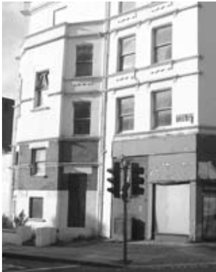
This elegant building at the corner of West End Lane and Finchley Road consist of a shop and 3 storeys of high-ceilinged residential space – currently occupied by pigeons.
